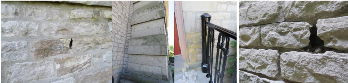
Variety of issues at the building including deep voids, cementitious mortar, organic growth and staining.
