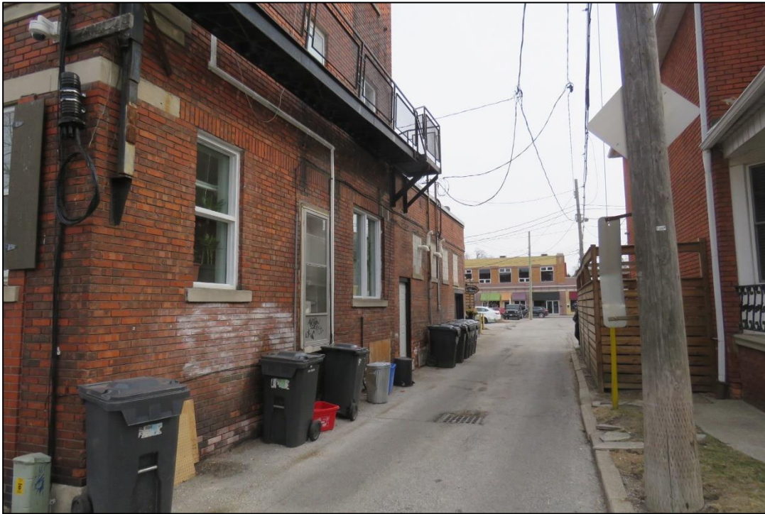
Figure 5 - Looking east towards east/west alley from Windermere Road (642 Windermere Road is on the right side of the alley)
