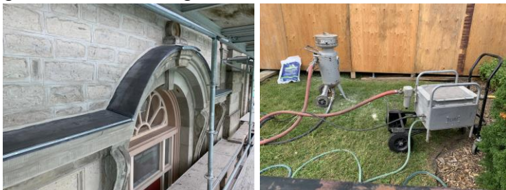
Lead coated copper flashing work above stone projections and the JOS & TORC Cleaning systems.
