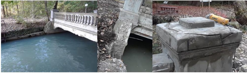
Photos of some of the visible deteriorated conditions of the bridge
