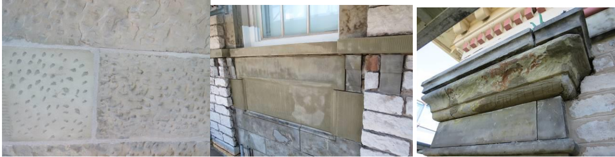
Jahn mortar repairs with appropriate texture and form to match and solid wood window sill repairs
